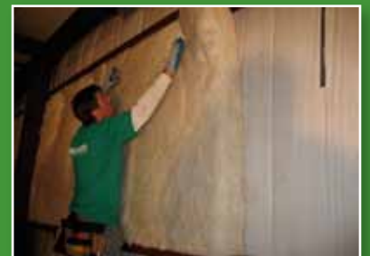
Insulation is cut to fit the full space and impaled on the Fast-R™ hangers.
